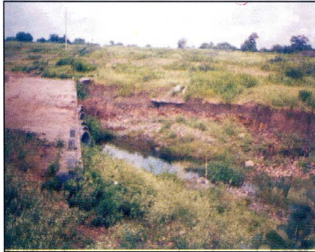
Plate 1. A view of side cutting of soil in Nallah due to heavy rainwater
